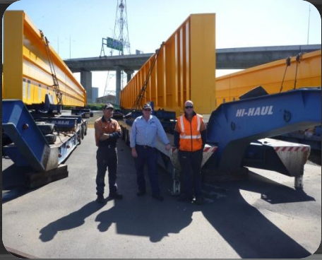
Photo of Dudley St bridge beams, Melbourne, with Staff: Danny Leones, Stuart Sutherland and Shane Duff, being installed weekend of December 16
